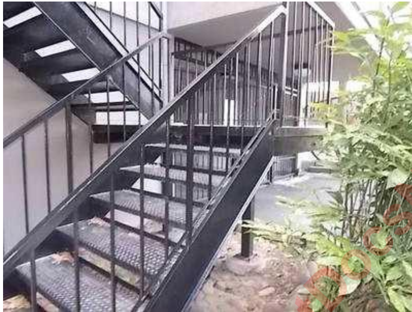
The Metal Stairway Replacement has been included in the Study. The Stairways are Painted by the Maintenance Supervisor and included in the Operating Budget.
