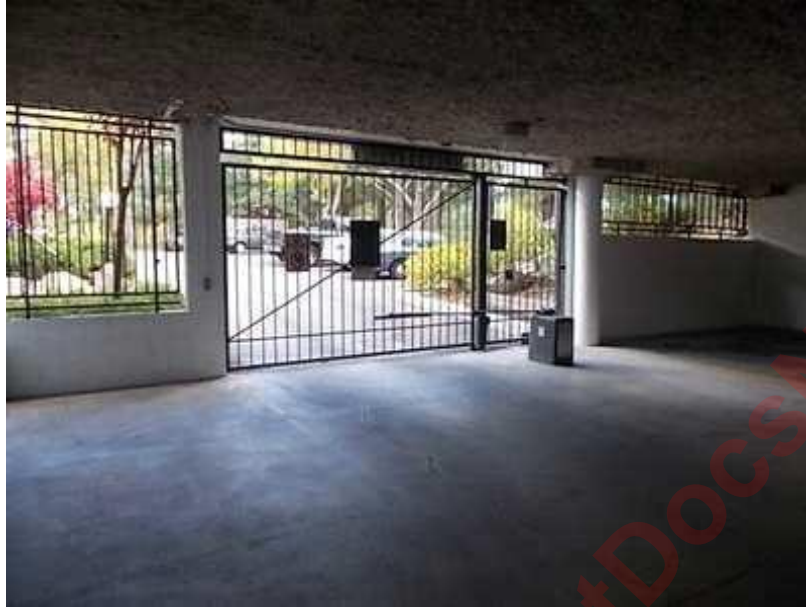
The Garage Entrance Components include the Gate and Gate Operator. There are 4 Entrance areas.
