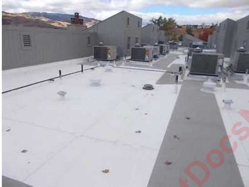
The Roof Replacement Schedule was provided by Scotts Roofing, Reno, Nevada. Each Individual Owner has their own HVAC System. These units are not maintained by the HOA.
