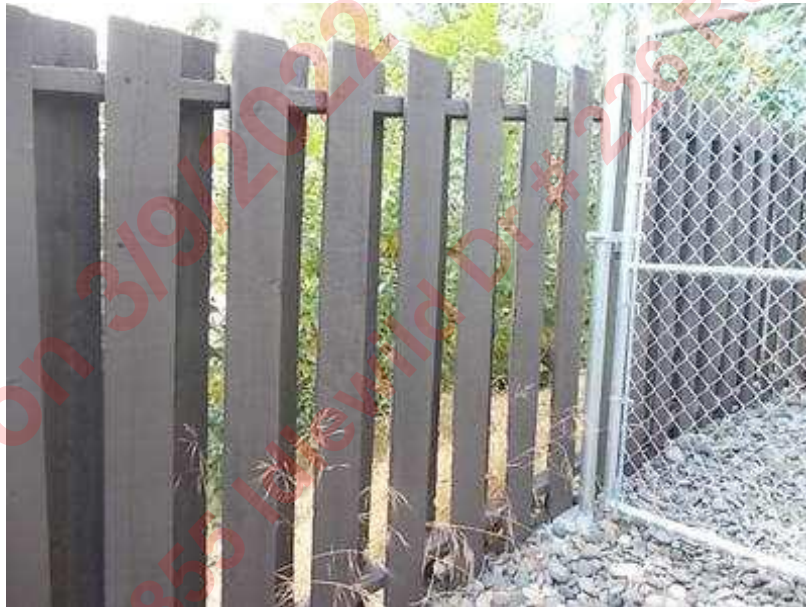
Repair and Painting of the Perimeter Wood Fence is done by the Maintenance Supervisor. This is a "good neighbor fence" shared with the adjacent property.
