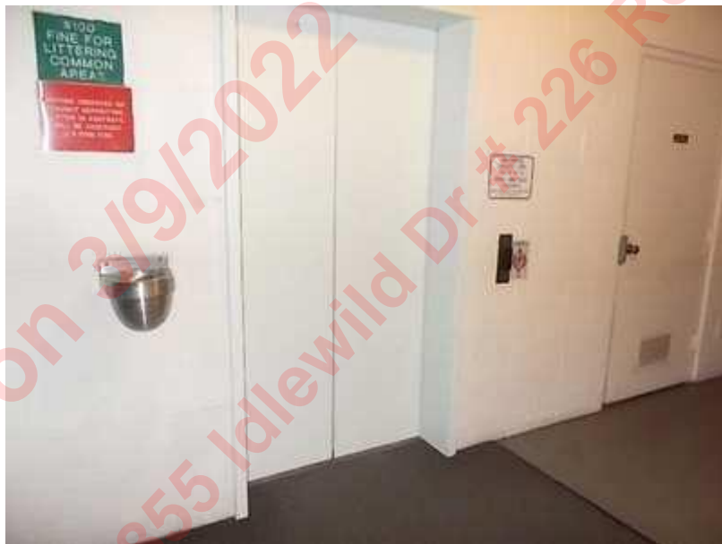
The Elevator Modernization Useful Life was obtained by Koch Elevators, Reno, Nevada.
