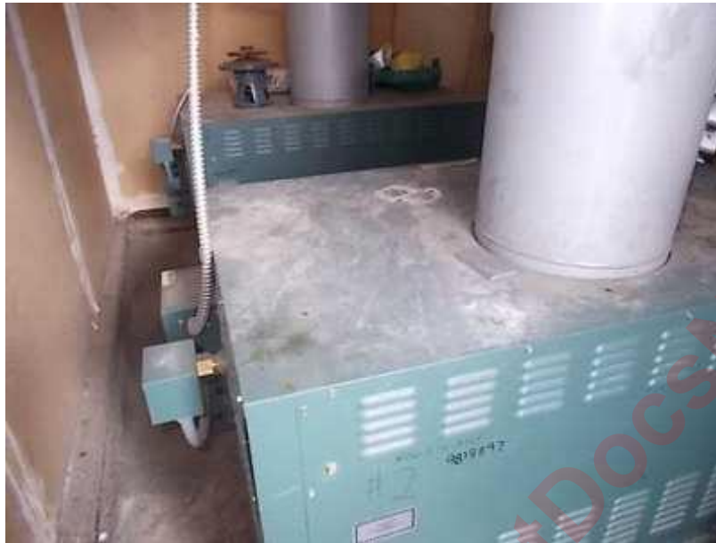
There are 2 Boiler Systems in building 2845. Replacement of the Boilers and Future Maintenance Costs were provided by Carl Michael Chinnici, Aardvark Mechanical, Reno, Nevada.
