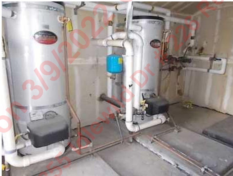
The 2 Water Heaters are located in Building 2855. These Units were installed in 2008 and have an Estimated Useful Life When New of 12-15 Years. Future Replacement has been included in the Study. The Replacement Cost and Estimated Useful Life was provided by Carl Michael Chinnici, Aardvark Mechanical, Reno, Nevada.
